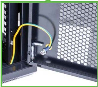
Door is grounded to the cabinet frame
