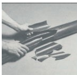
Remove damaged or faulty ducting
